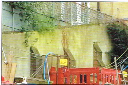
Actually, at time of writing, these Grade II listed buttresses have disappeared under a huge mound of sand.
